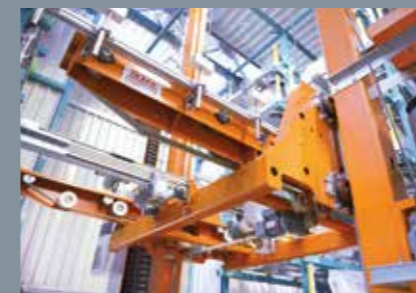
Storage and retrieval machines
